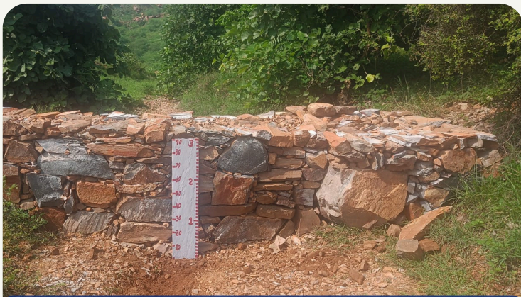
Gauge installed on the upstream side of the structure to monitor silt deposition under DLT works.
